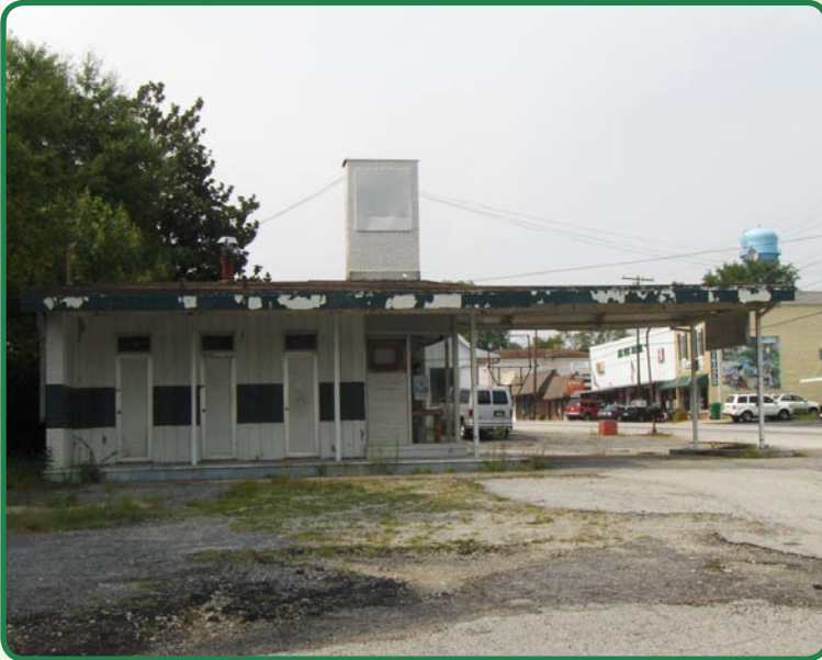
Aging gas station building at corner of Main and Thornton Streets in Downtown Palmetto
